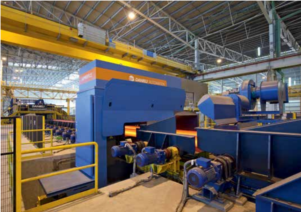
HiPROFILE typical plant installation
